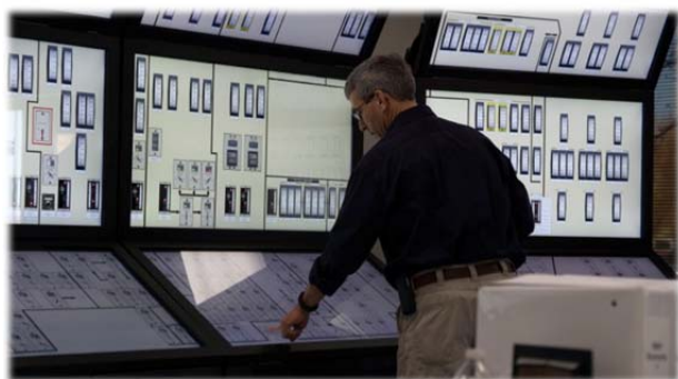
FIGURE 1. Touch screen benchboard panels.
