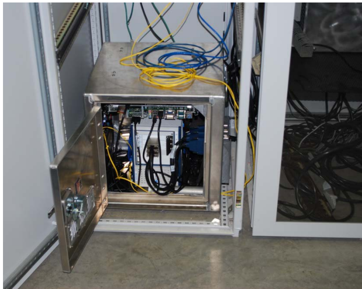
Figure 2. INL Typical Substation GMD Data Acquisition System.
