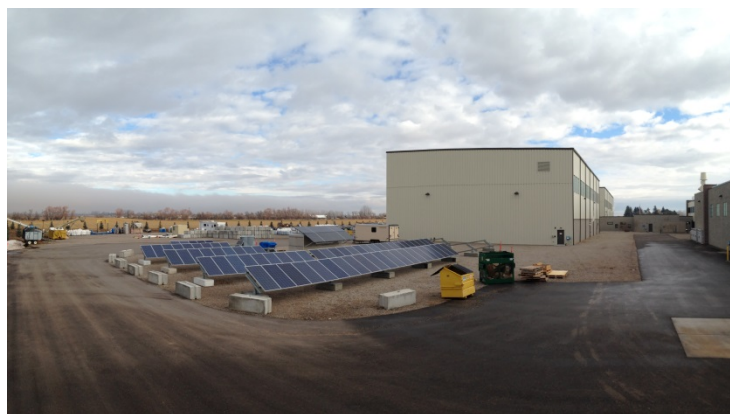
Figure 1. Portions of INL microgrid research assets.
