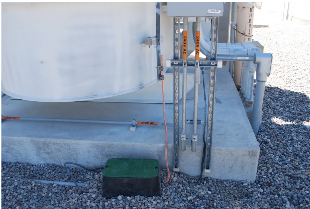
Figure 2. Typical INL transformer—GMD ground current measurement.
