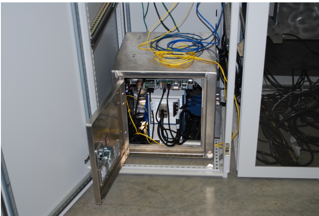
Figure 3. INL typical substation GMD data acquisition system.
